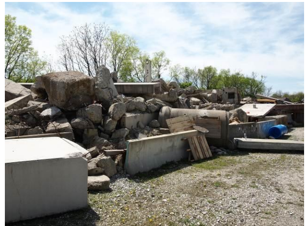
Fig. 2. Rubble pile at OH-TF1 Training Center
